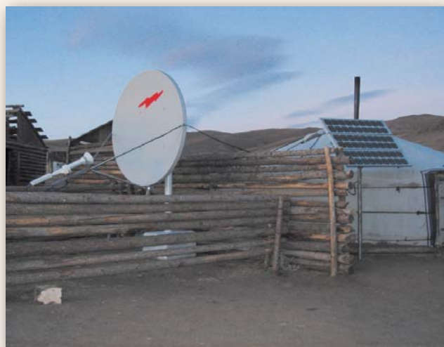
GPOBA funded telecom infrastructure in Mongolia.
